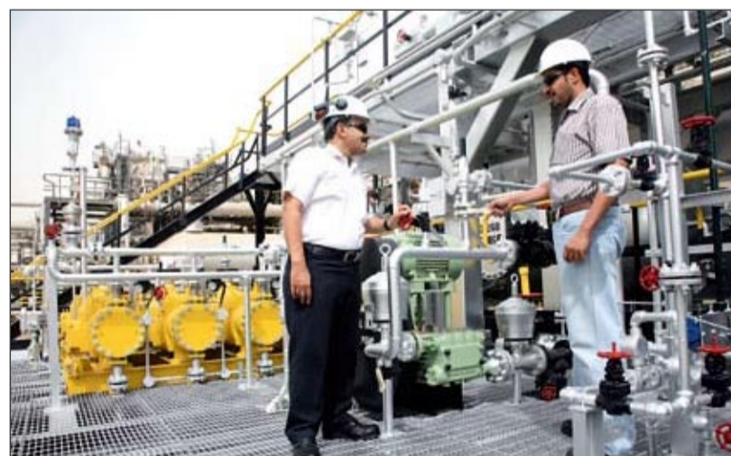
Rashid M. Shammari, left, speaks with plant console controller Ibrahim M. Shahrani as they stand upon the safety simulator in front of Gas Plant No. 462.
